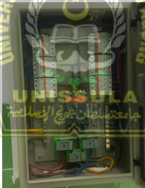
Gambar 4. 2 Panel SDP Lantai 2 ( Sub Distribution Panel)
