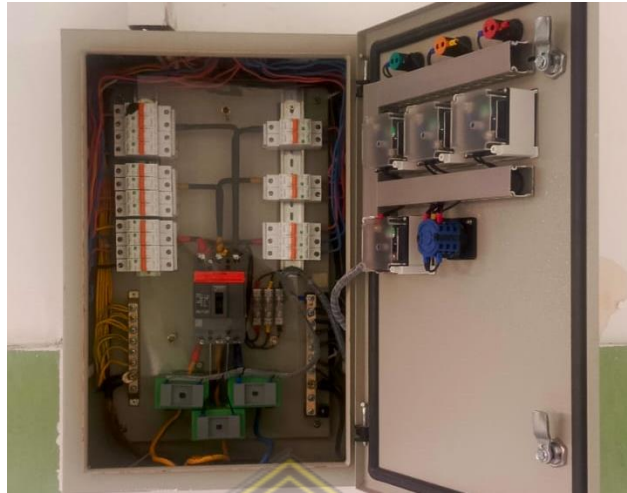
Gambar 4. 1 Panel SDP Lantai 3 (Sub Distribution Panel)
