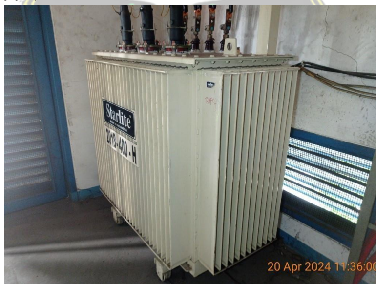
Gambar 2.16 Transformator Distribusi 20 kV
