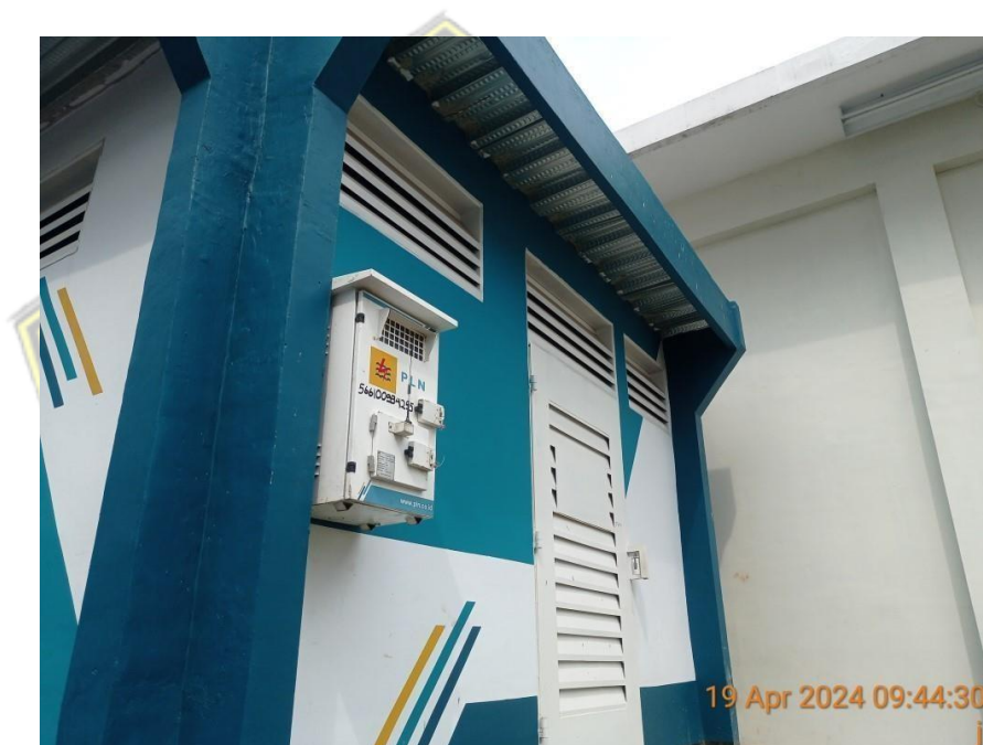
Gambar 2.4 Gardu Distribusi ( Gardu Beton )
