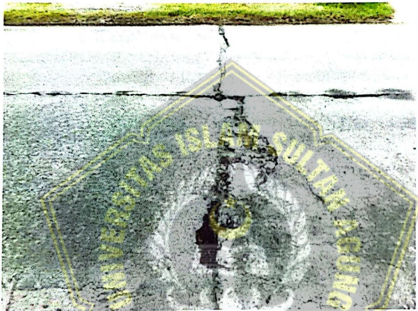
Gambar 4.14. Retak daya tahan ( Durability "D" Cracking )
