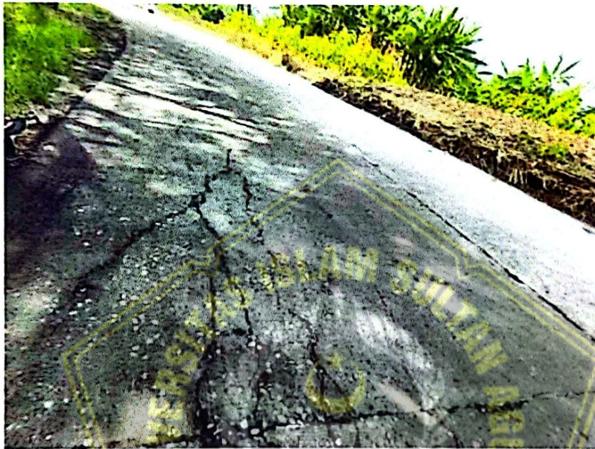
Gambar 4.11. Retak slip ( Slippage Cracking )
