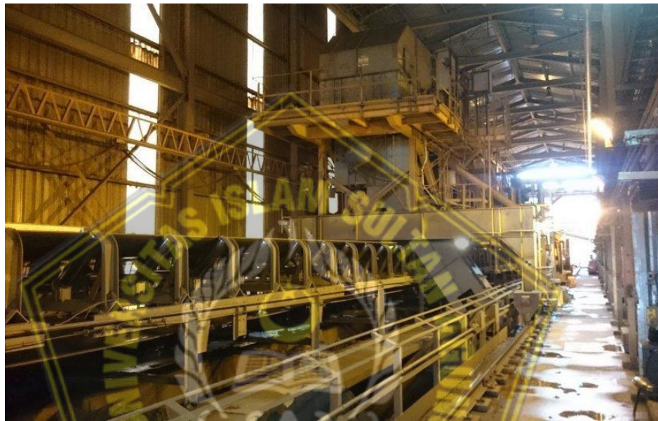
Gambar 2. 17. Tripper Car PLTU Tanjung Jati B unit 1 & 2
