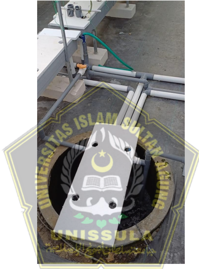
Gambar 3.4 Penampakan Reservoir di Greenhouse
