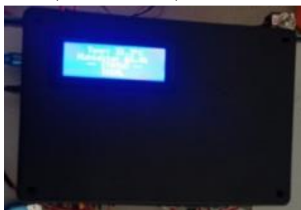
Gambar 5. 2 Panel kontrol sistem
