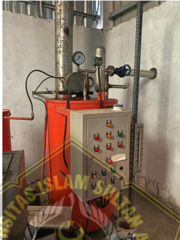
Gambar 4.16 Mesin Boiler PT. Sinergi Brebes Inovatif
