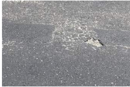
Gambar 4. 25 Kerusakan Lubang STA 1+820-1+8700 (Sumber: Hasil Survey 16-10-2023)
