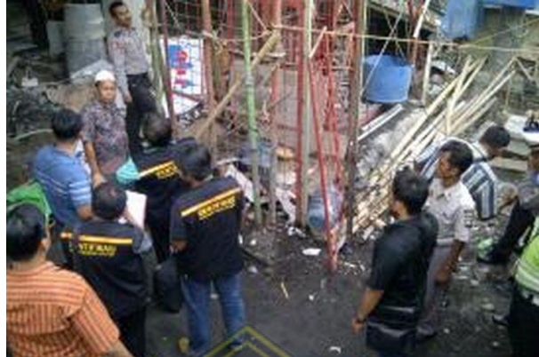
Gambar 4.23 Terjepit Bekisting/ Scaffolding
