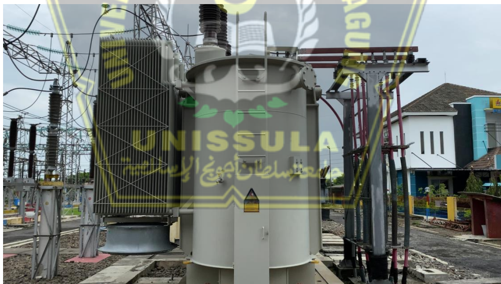
Gambar 2.14 Transformator Tenaga 60MVA GI Krapyak
