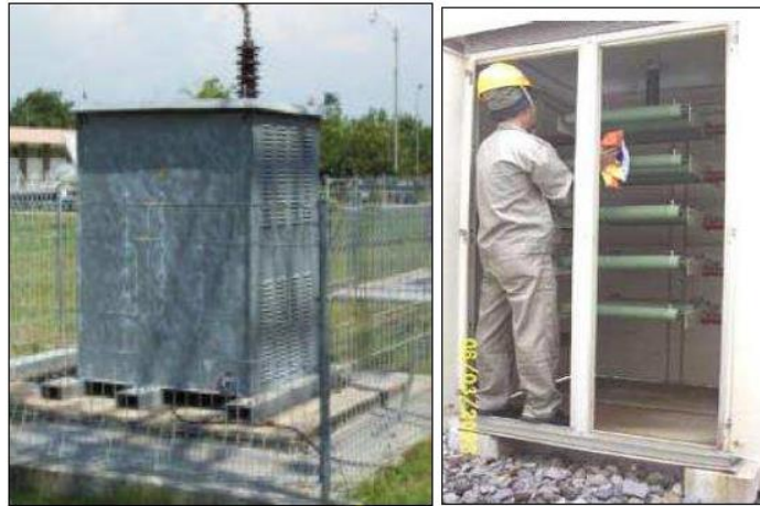
Gambar 2. 23 Netral Grounding Resistor (NGR)
