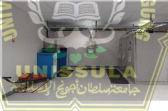
Gambar 2.1. Main Distribution Panel (MDP)
