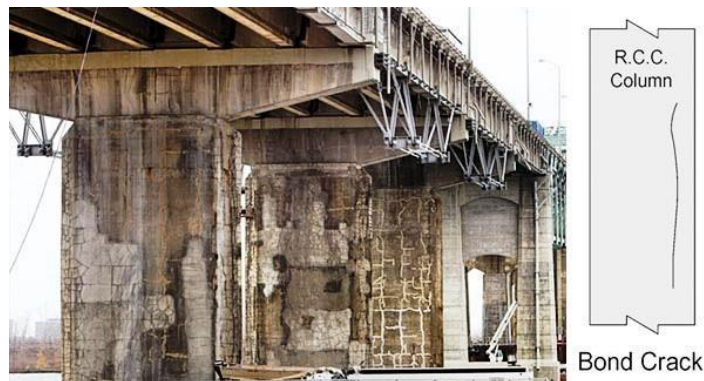
Gambar 2.4 Retak Korosi ( Corrosion/Bond Crack )
