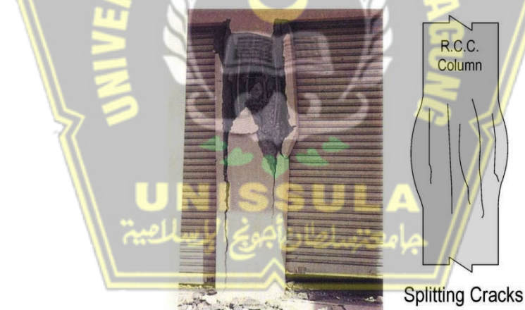
Gambar 2.3 Retak Pecah ( splitting Crack )
