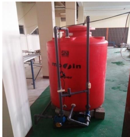
Gambar 3.16: Pompa Pengisian Air
