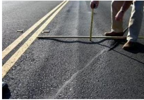
Gambar 2. 6 Slip ( Slippage Cracks )
