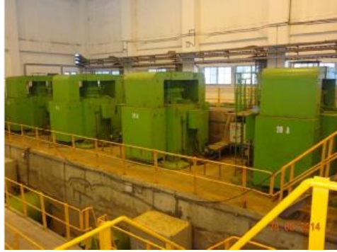
Gambar 2.2 Circulating Water Pump
