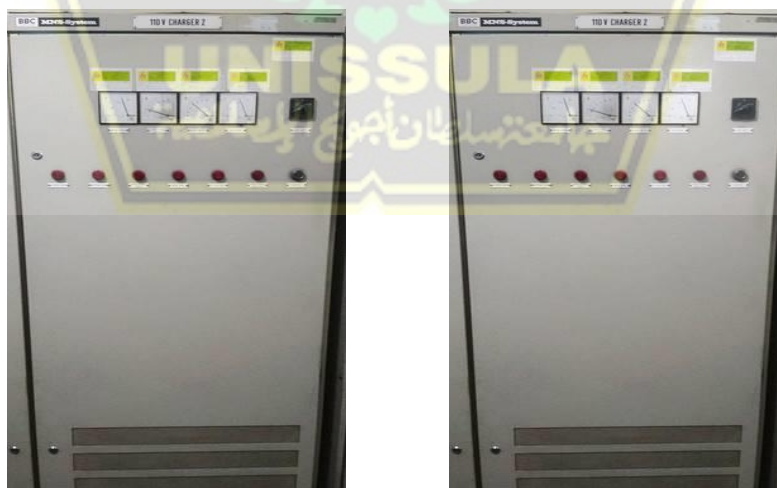
Gambar 3. 2 Charger Unit 1 & 2 110V GI 150 kV Spondol
