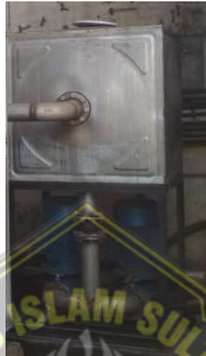
Gambar 4.8 Water pumping unit
