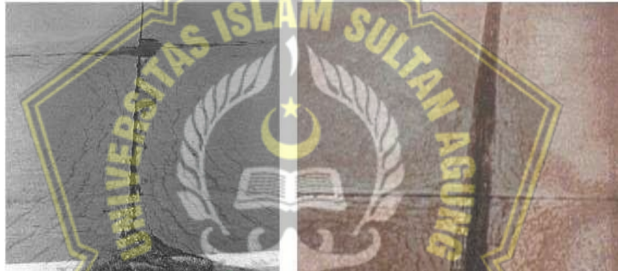
Figure 6.13. Examples of Durability Crack in a Slab [18]
