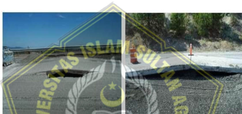
Figure 6.21. Examples of Blowup Distress
