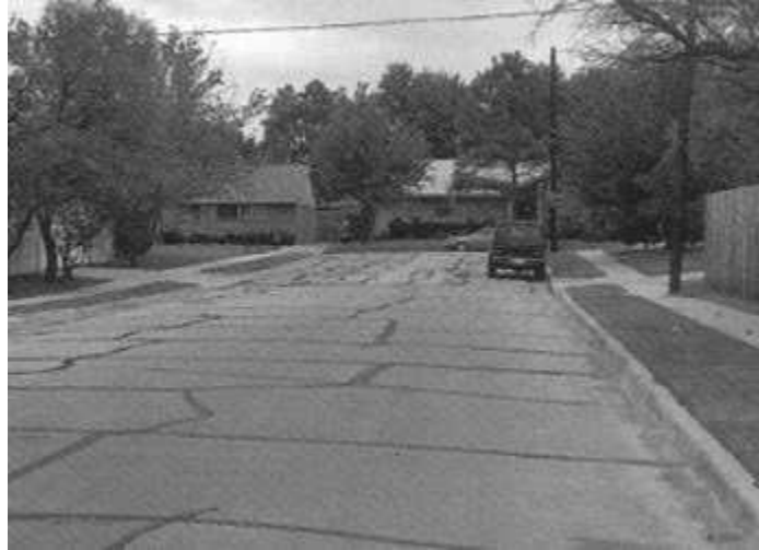
Figure 6. 7. Swelling in Flexible Pavement
