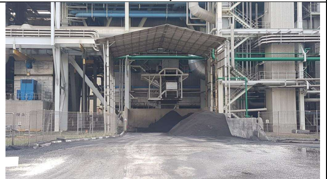
Bottom ash Bunker Unit 3
